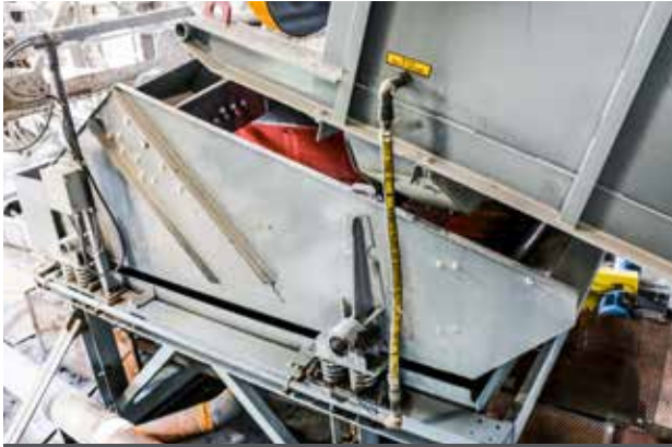
RECYCLE WATER LINE
